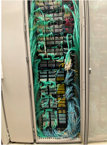
Figure 6: The rack (nr. 16) with all the fiber cabling in the DC1.
