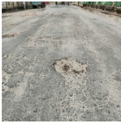
(a) Sample 1 (Pothole)
