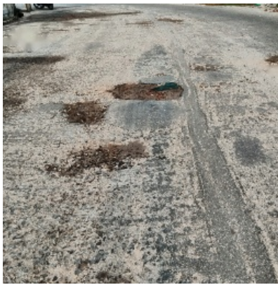
(b) Sample 2 (Pothole)
