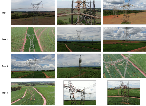
Figure 3: Sample of images of each task for the TAESA Transmission Towers Dataset.
