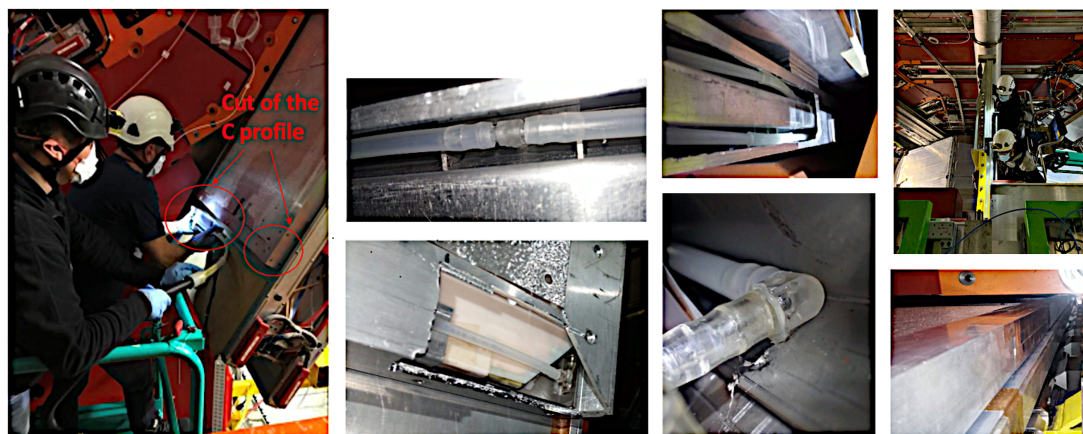
Figure 70: Photographs illustrating the gas-leak repair procedures. Left: scientists working on the repair procedure. Middle left: access to broken component. Middle right: repairing of components. Right: closing and validation.
