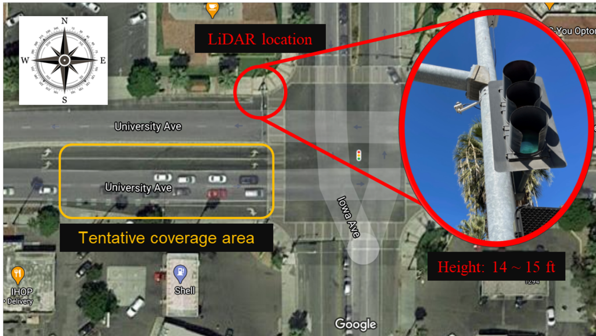
Figure 5: Location and installation of the equipped roadside LiDAR.
