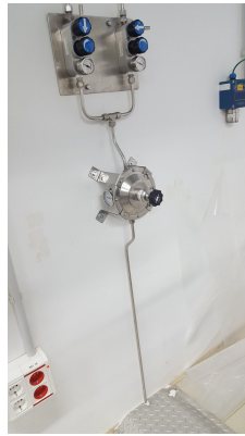
Figure 22: ATEKO-Air main line in Hall C.
