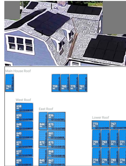
Figure 1: A residential solar array (top) with 31 panels deployed on four roof planes, and real-time panel-level generation data from the array (bottom)
