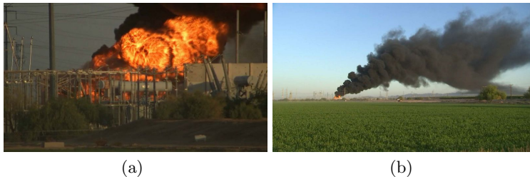
Fig. 1. Transformer fire at Salt River Project (SRP)’s Rudd substation in Avondale [7].
