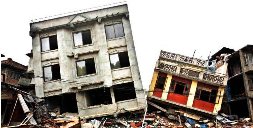
Figure 1. Plastic “hinging” of foundation due to the rocking mechanism in Kathmandu Valley, Nepal as a result of the M_w 7.8 2015 Gorkha earthquake (Hume, 2017).
