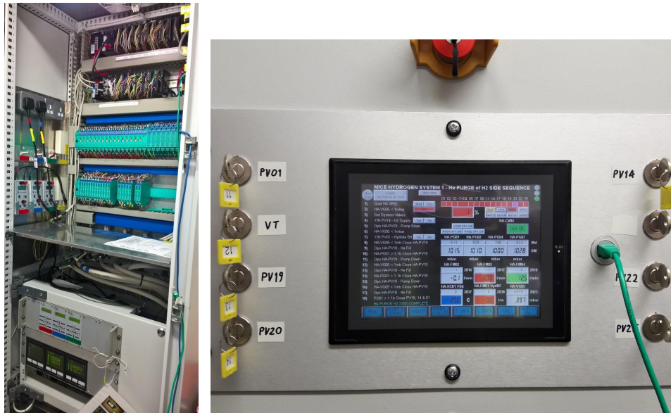
Figure 17. Photographs of the H 2 -system control cabinet (left), and the touch-screen panel (right) between the keyed over-ride switches and below the emergency shut-down button.
