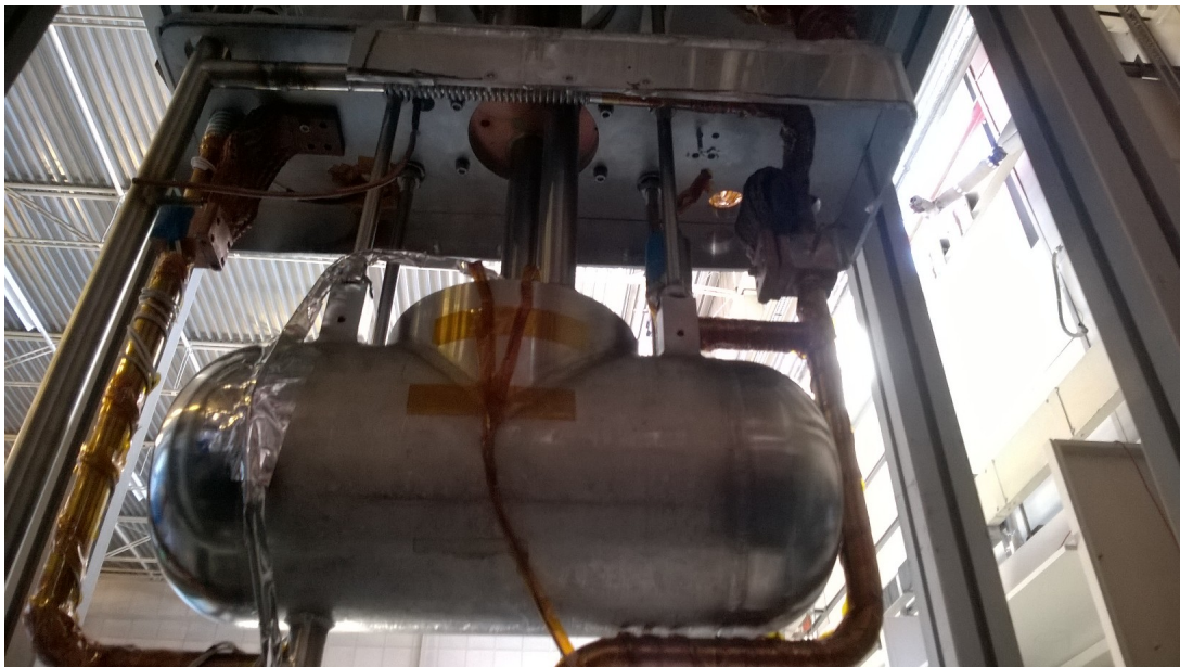
Figure 14. Photograph showing the condenser with the bypass loop added. The aluminium thermal shield had been cut away for this modification and was re-welded for the following runs.
