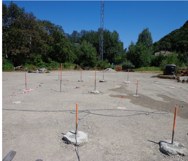
Figure 8: Photo of a soil reinforced with columns of concrete 0.4m in diameter and 15m in depth (Courtesy of Ménard).
