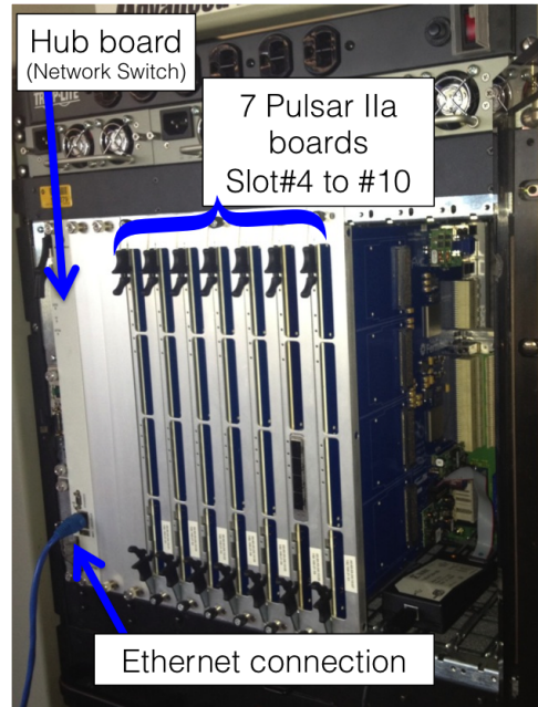
Fig. 11. Our 14 slot ATCA shelf with a commercial switch blade in slot 1 and seven Pulsar IIA boards in slots 4 through 10.
