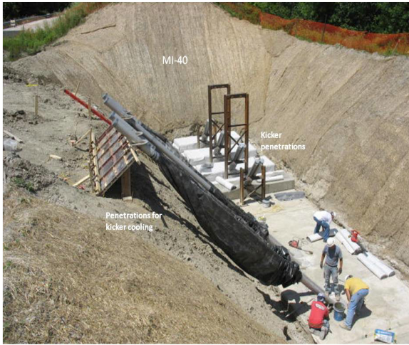
Figure 2: Installation of new kicker penetrations. The shielding has been removed to expose the Main Injector tunnel ceiling. Note gray penetration pipes.
