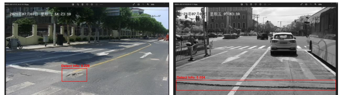
(c) Small pothole with big DetectInfo value (d) Big patch-crack with small DetectInfo value
