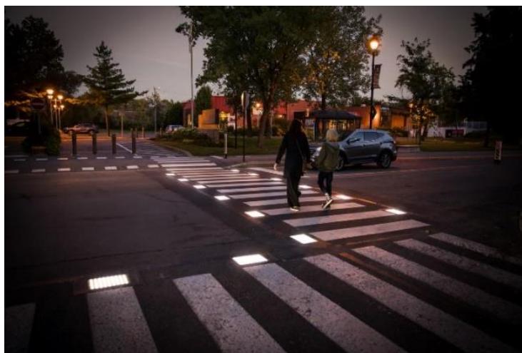
Fig. 6. A newly installed lighting system in Candia, Quebec, Canda, for improving intersection traffic safety [Source].
