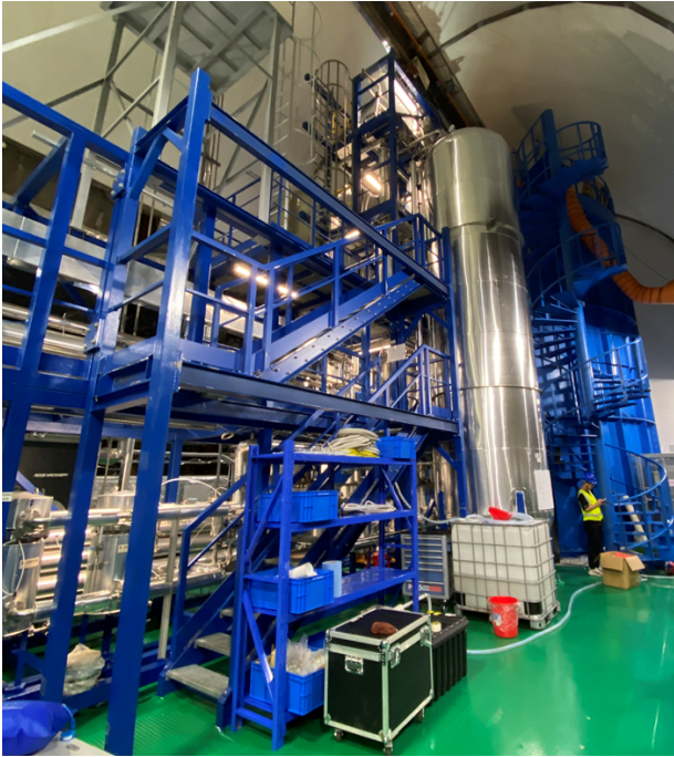
Figure 6: Stripping plant installed in the Underground LS Hall at JUNO site.
