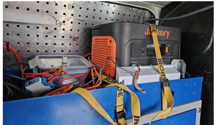
Fig. 4: Raspberry Pi, relays, connections to car battery and ignition, Jackery Explorer 2000 Pro with smart Zigbee socket and Starlink FHP dish power supply.
