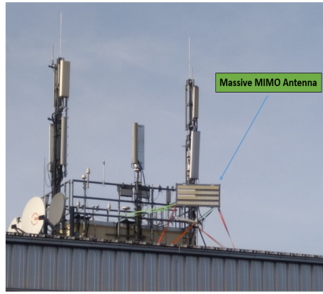
(b) BS antenna with 64 antenna elements is shown here.
