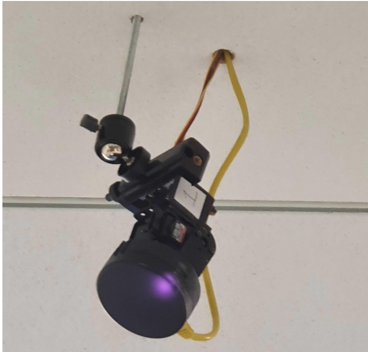
Figure 5: LiFi Antenna mounted on Pan-Tilt servos and connected to RaspberryPi in ceiling.
