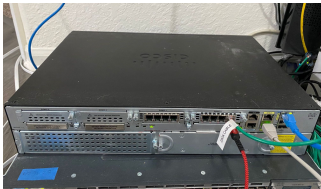
(a) Cisco 2911 as VoIP server/gateway and a tunnel endpoint
