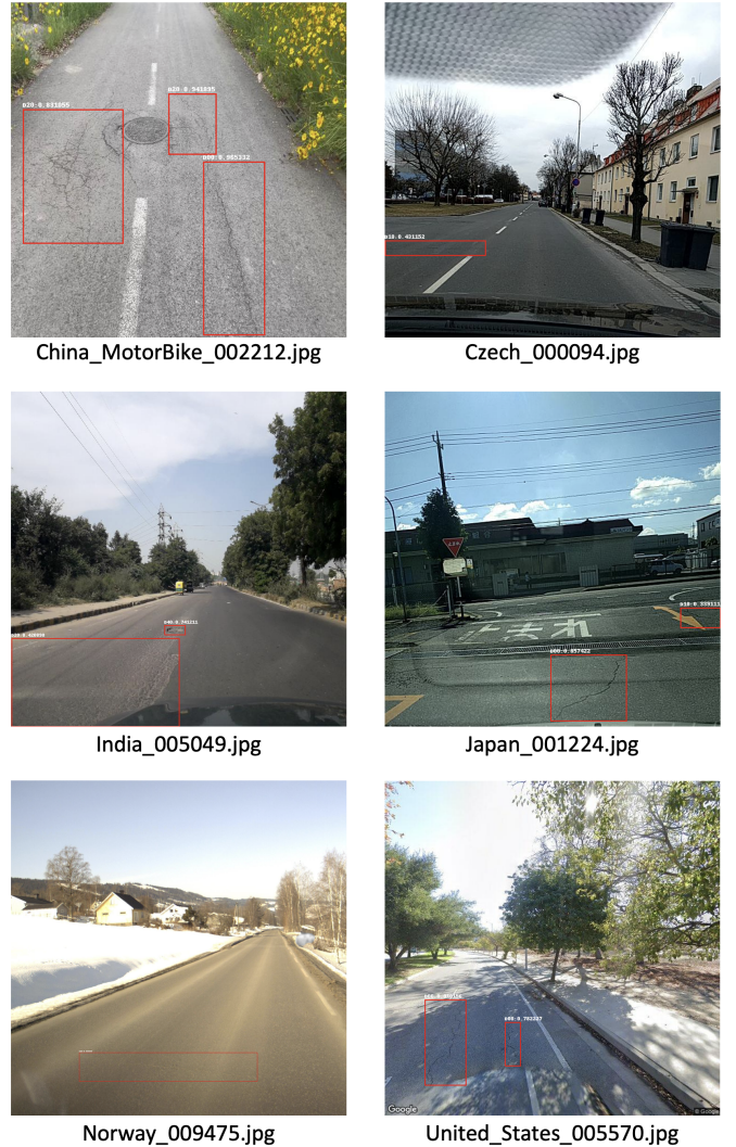
Fig. 9. Examples of damage detection from road images using the approach proposed in this paper.
