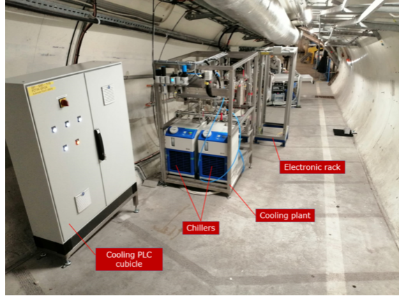
(b) Detector services upstream in TI18
