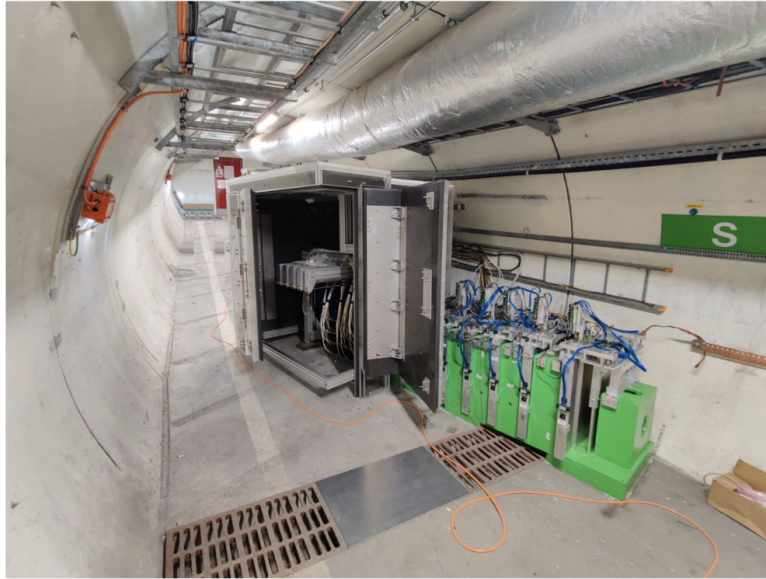
Figure 53: Global view of the detector in TI18 after the installation of the neutron shield.
