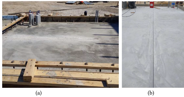
Fig. 12. Pictures of Pour 2. (a) the foundation. (b) the saw cut made into the foundation.
