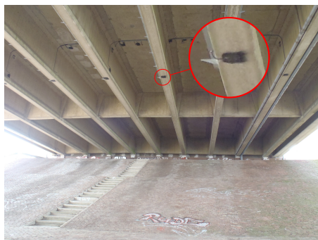
Fig. 3: Picture that highlights the placement of the sensors that are attached to the girders and bottom of the deck (from (Miao 2014)).
