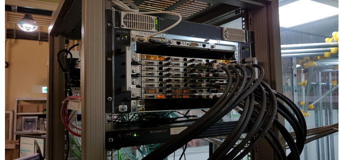
Fig. 1. Front view of the DHH system. In this ATCA shelf, four DHH carrier cards are installed and connected with CameraLink cables, attached to the DHIs, to the detector.
