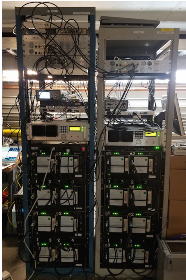
Figure 6. VLBI backend installed at the SPT control room. These racks comprise a 64Gbps data recording system.
