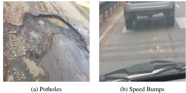
Figure 1: Road surface conditions in Nairobi (a) Potholes (b) Speed Bumps.
