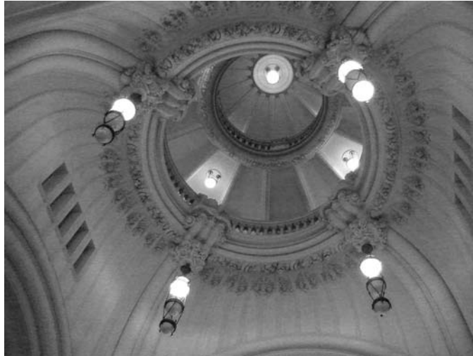
Figure 8: Central vault as seen from the ground floor of the Barolo Palace.
