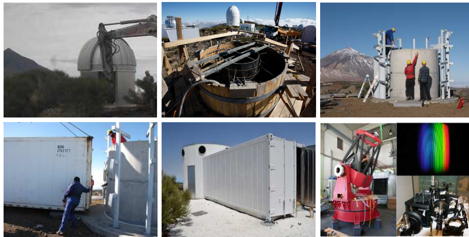
Fig. 1 The evolution of SONG-OT between October 2010 and September 2011 (timeline from left to right, from top to bottom): the removal of the STARE telescope, the construction of the dome support and container, the telescope, the spectrograph, and an example of the échelle spectrum.
